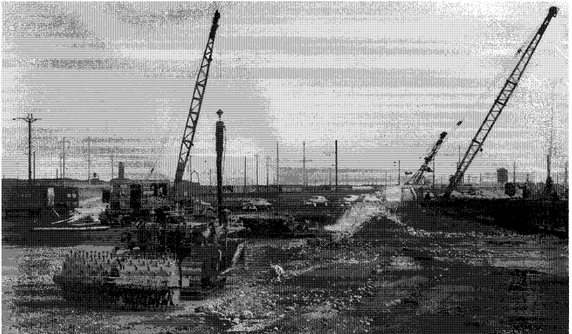
Ground breaking at the South Kearny Rail Yard in New Jersey for the Pennsylvania Railroad, taken 1 January 1955 looking eastward.
