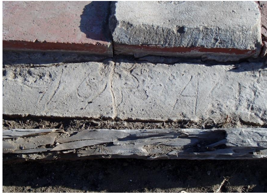
Figure 23. Illegible writing on the concrete collar.
