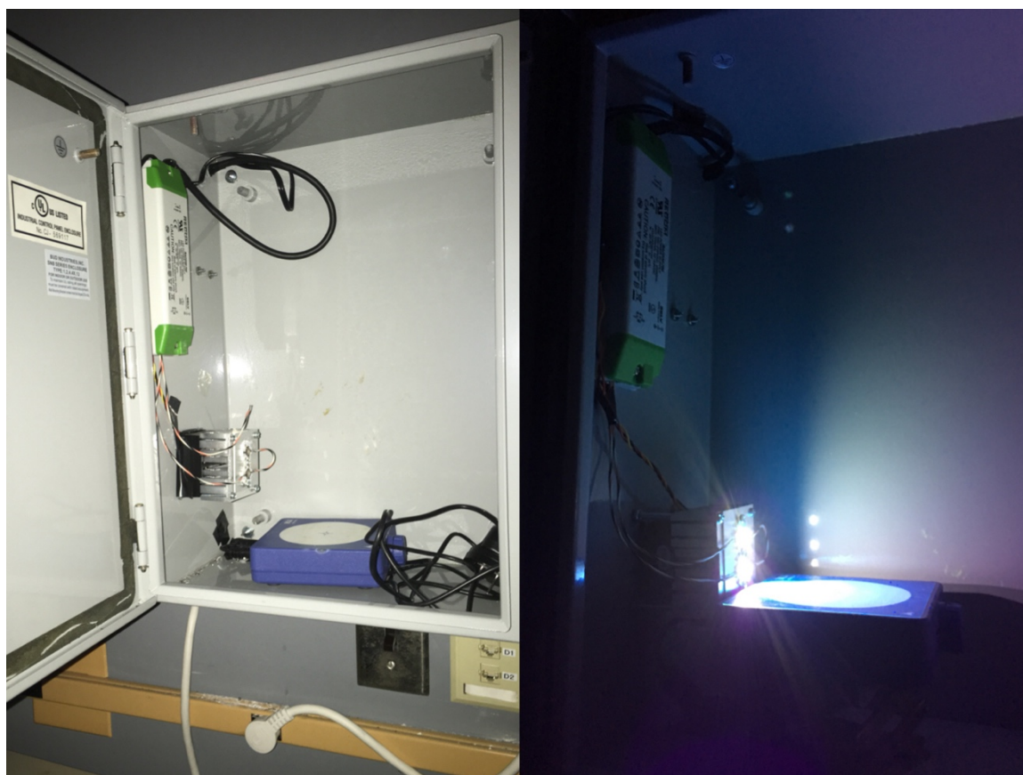
Figure 3.12 Steel electrical junction box equipped with UV LED irradiators
