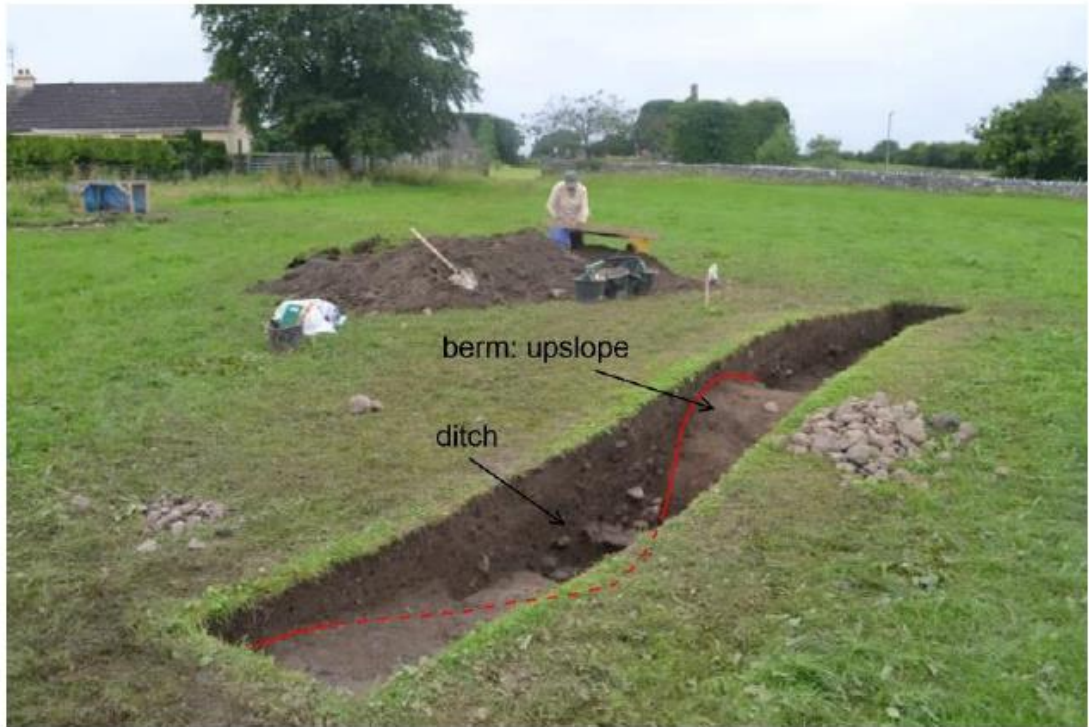
Figure 26: Excavation unit across a French drain composed of a berm and ditch (Conyers 2018: 86).
