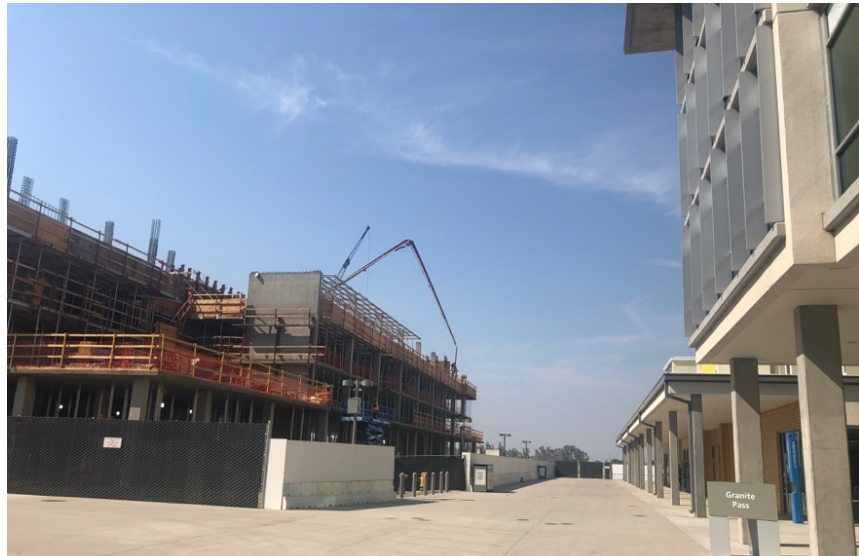
Figure 10. On the right is Granite Pass building and to the left is building construction for the second delivery in Fall 2019
