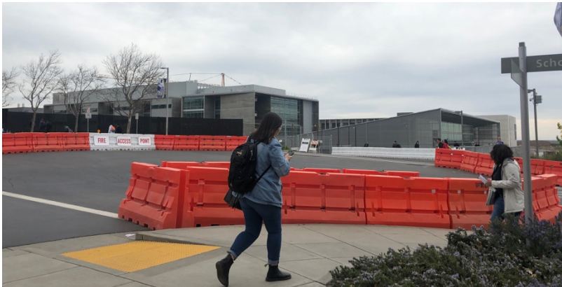
Figure 36. Top of the hill right before the start of the bridge has been blocked by construction barriers
