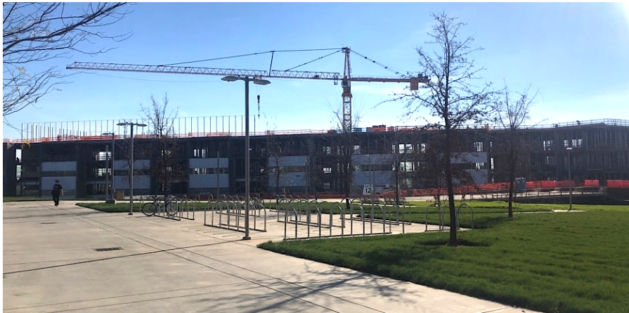
Figure 14. Construction of the second delivery phase, scheduled to be complete by Fall 2019
